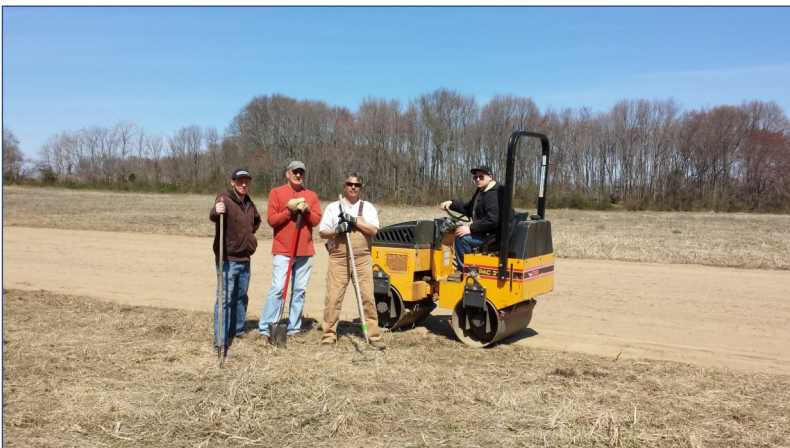
In 2014, a hard working and energetic bunch of individuals installed a fabric runway at Pulda Farms. Pictured above are just a few of the guys, (Left to right) Chris Orban, Gerry R. Mike D and his son Joey on the roller.
